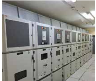
JAM: Breaker for new Transformer
